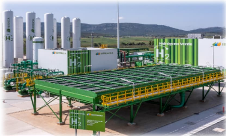
20 MW Green H2 plant in Puertollano
