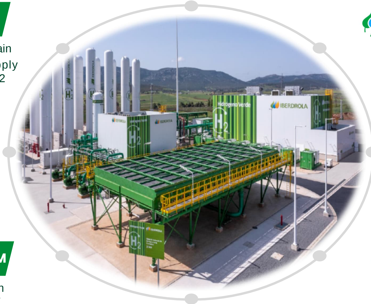
Puertollano 20 MW plant One of the largest electrolyzer in Europe, operating since 2023
