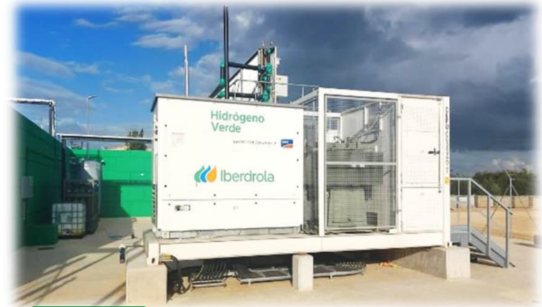
1.25 MW Green H2 plant in Benicarló
